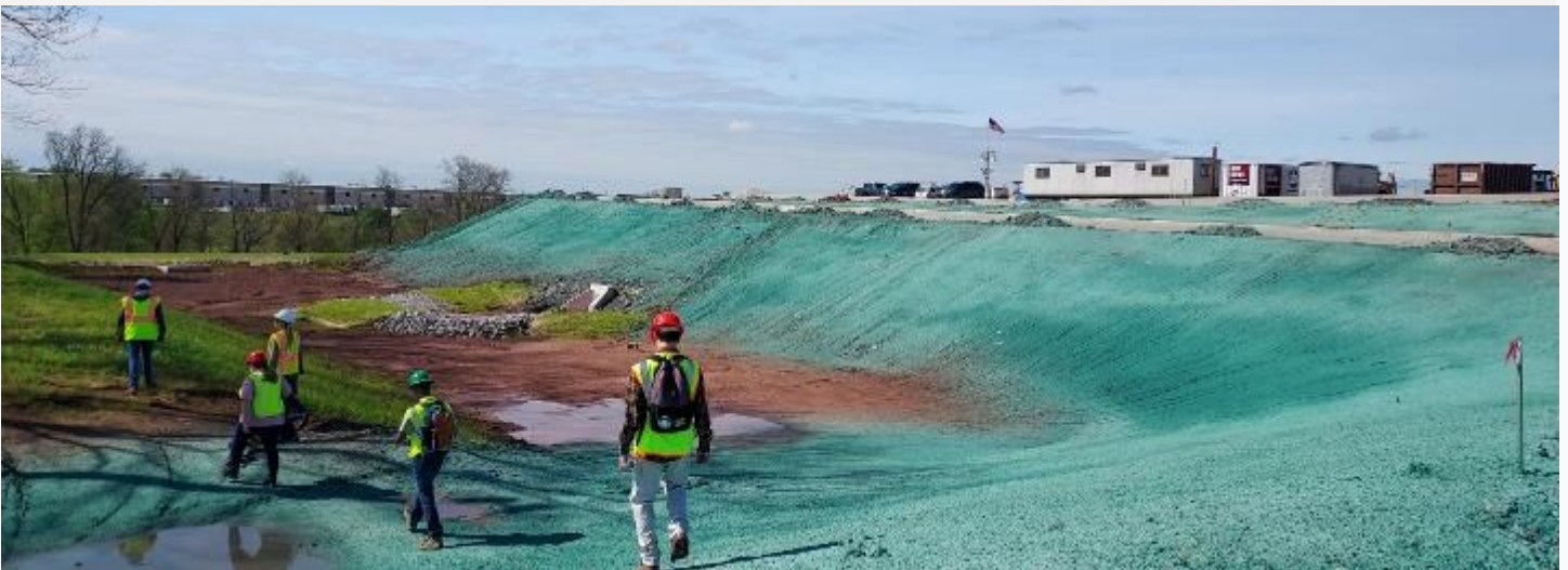
Above: Participants tour a large construction site. The slopes were freshly hydro-seeded, making the area look otherworldly.
