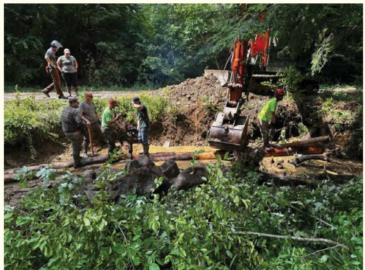
In the photo above, a crew can be seen installing a mudsill earlier this summer.
